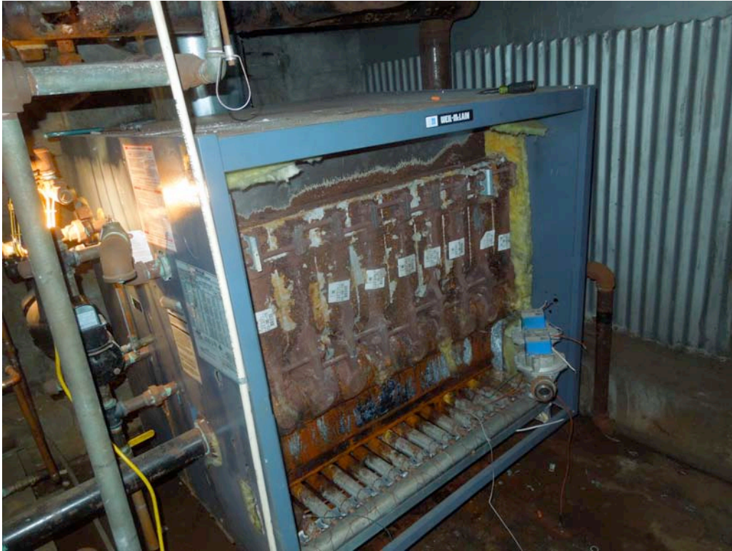
This is the inside of the old boiler. Notice the rust and corrosion.
