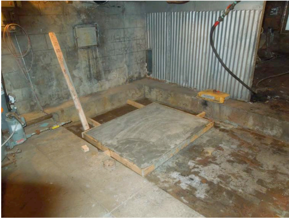
A cement platform has been poured, ready to receive the new boiler next week.
