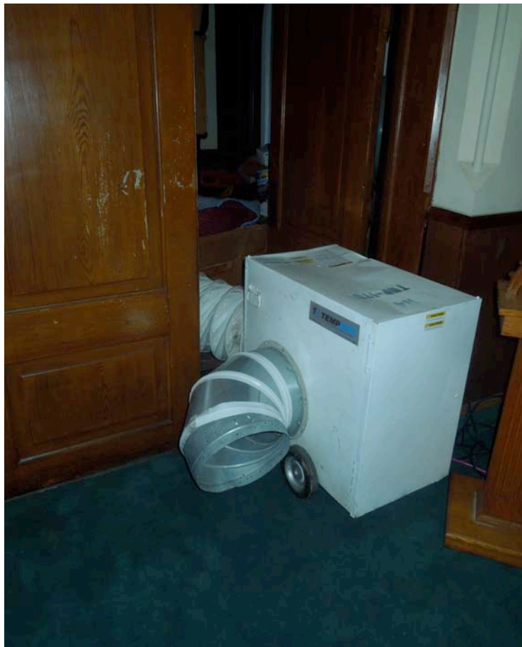
In the meantime, this is the gas space heater to heat the chapel. It works! The temperature in the chapel for Mass this morning was 68 degrees.
