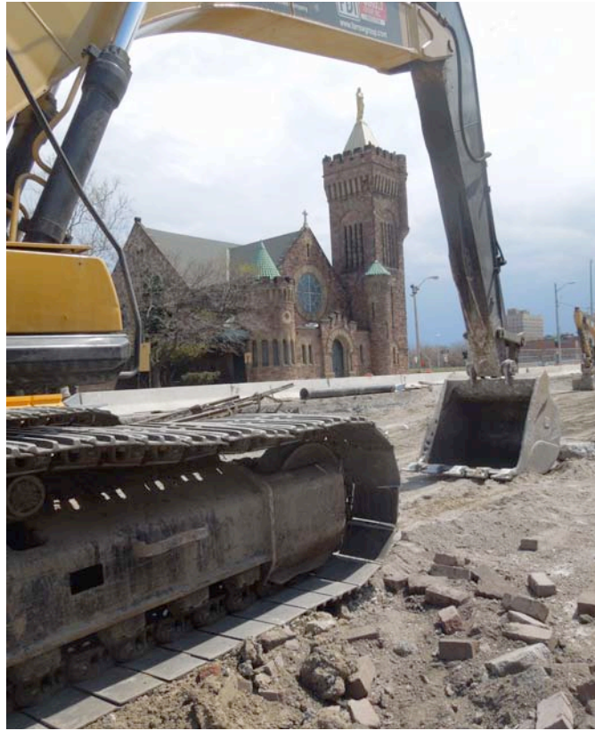
Attach of the Earth Movers! As the M-1 light rail gets closer, it looks like Rosary will be gobbled up!
